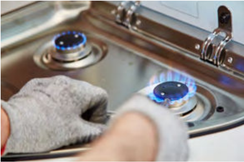
Test on operation of the gas pipes.
